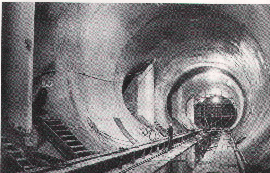
The power tunnel which carries water from Lake Gordon into the underground hydro-electric power generating system
